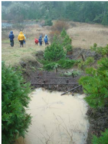
(A brush check-dam built adjacent to an orchard site to repair a badly incised gully.)
